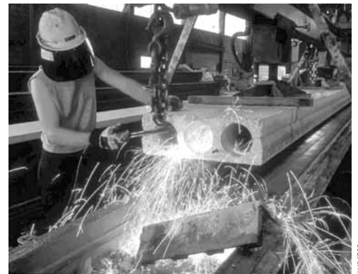
A Strescon worker cuts the end of a prestressing strand from a precast hollow-core plank. The plank is formed by pouring concrete into a form and vibrating it to consolidate the concrete. The vibrator is lubricated with Molykote® BR2-Plus Multi-Purpose E.P. Grease.
